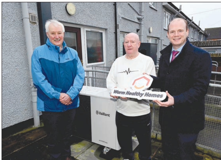
Communities Minister Gordon Lyons (right) pictured at the launch of the Warm Healthy Homes Strategy in Belfast with (left) John McMullan, Vice Chair, Northern Ireland Housing Executive; and householder Trevor Rainey, who had a Low Carbon retrofit upgrade fitted to his home by NIHE last summer.
